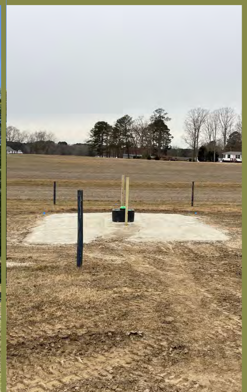
A newly installed livestock watering system providing clean drinking water for horses and helping to keep sediment and nutrients out of waterways.
