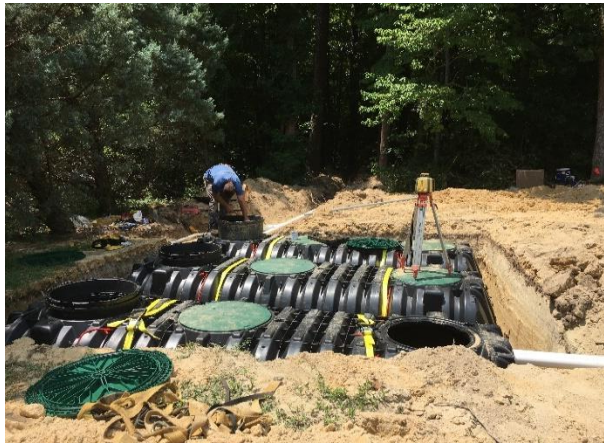
Underground Detention Tanks
