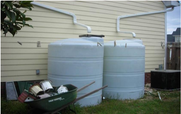
Rain Barrels with Roof Drains
