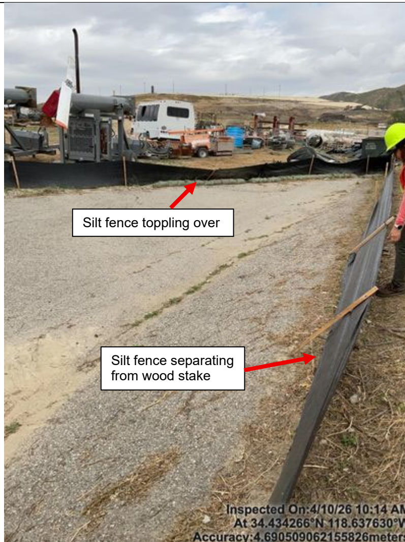
Photo 33 Silt fence with improper installation in need of repair.
