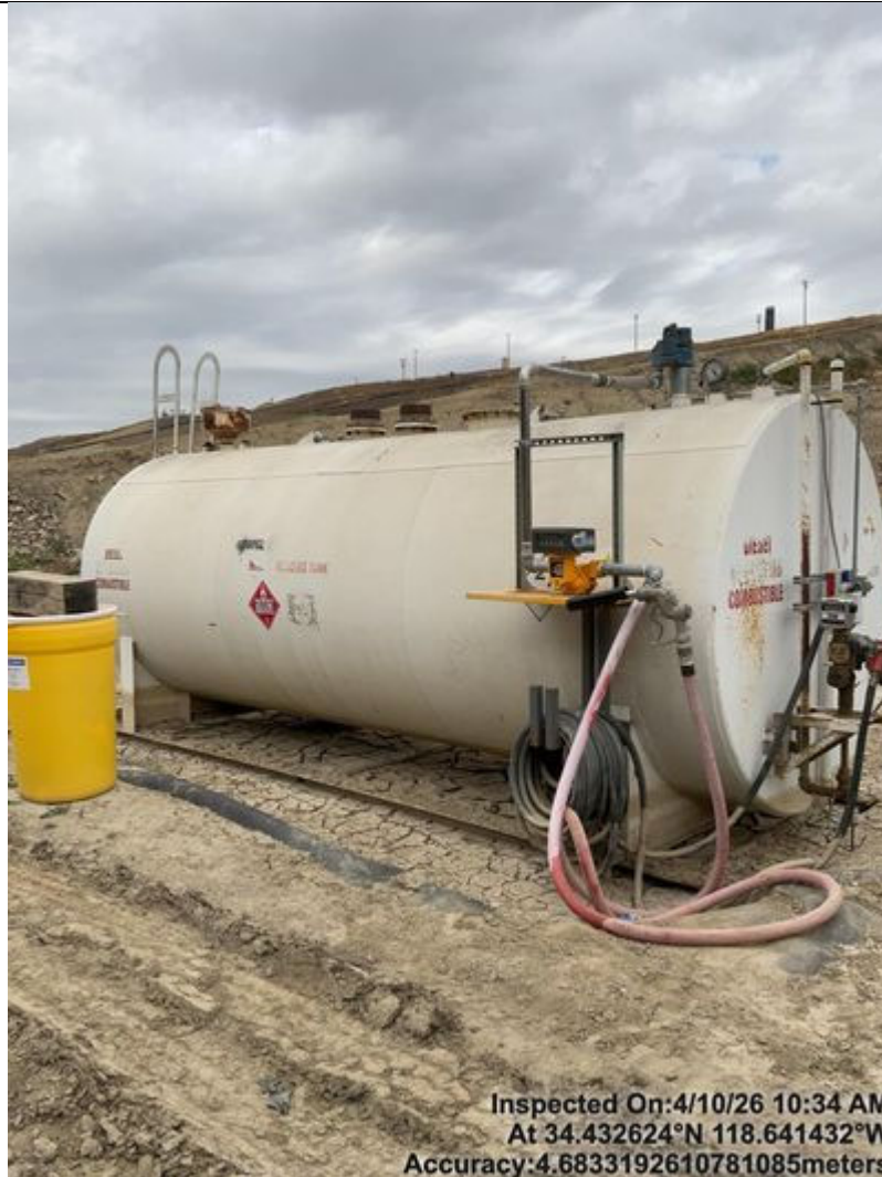
Photo 64 Diesel storage tank and fueling area
