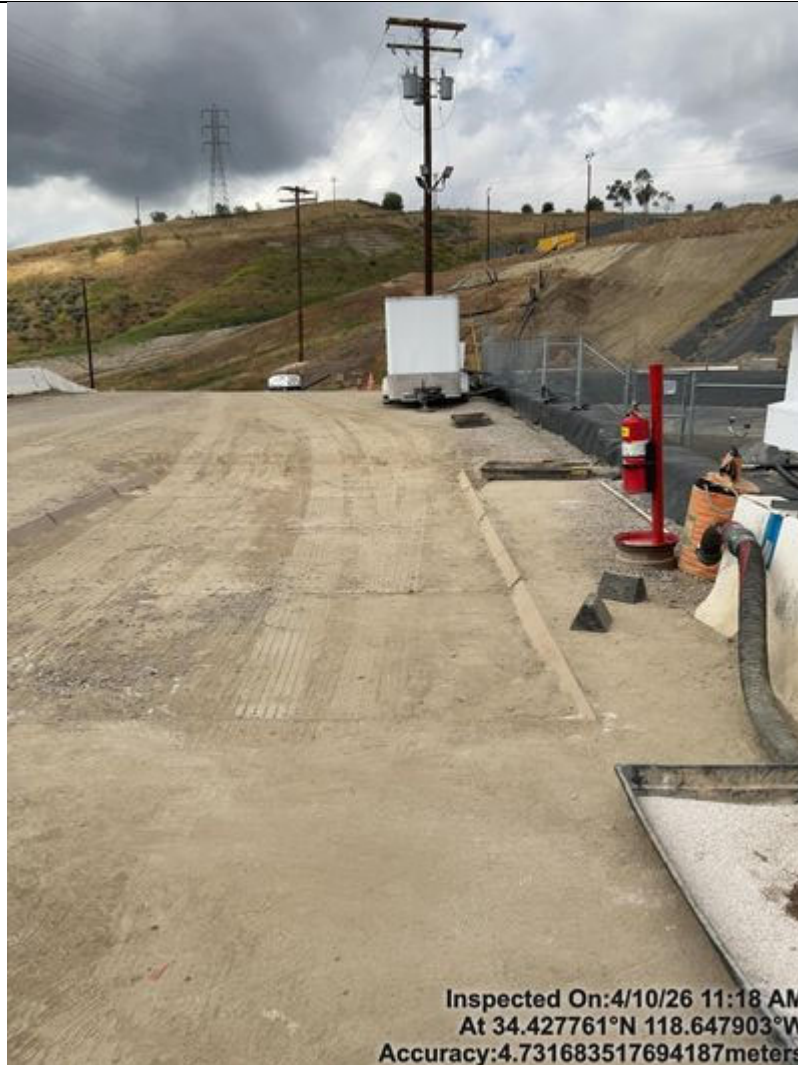
Photo 96 Loading pad for loading treated leachate into trucks
