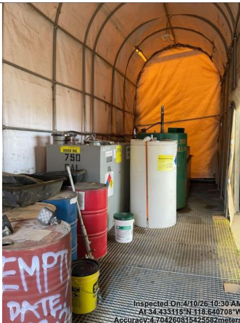
Photo 57 Covered oil storage with secondary containment
