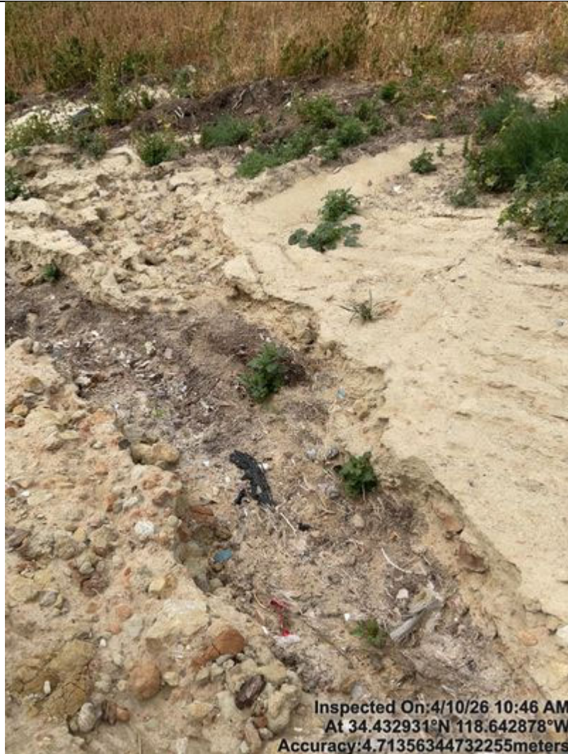
Photo 77 Close up of erosion next to the erosion control BMP
