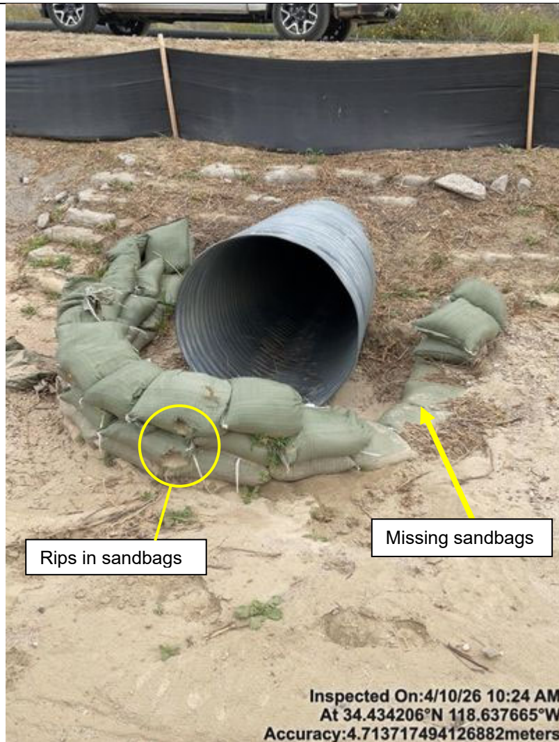
Photo 39 Close-up of culvert with sandbags in need of repair
