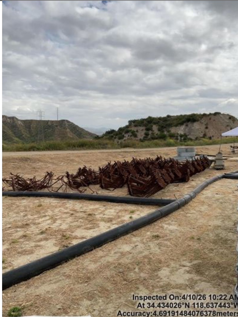
Photo 51 Metal material stored outdoors. I observed rust on the metal material
