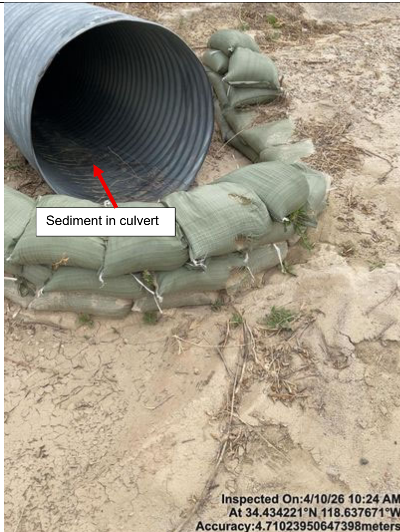
Photo 41 Close-up of sediment buildup and missing/torn sandbags
