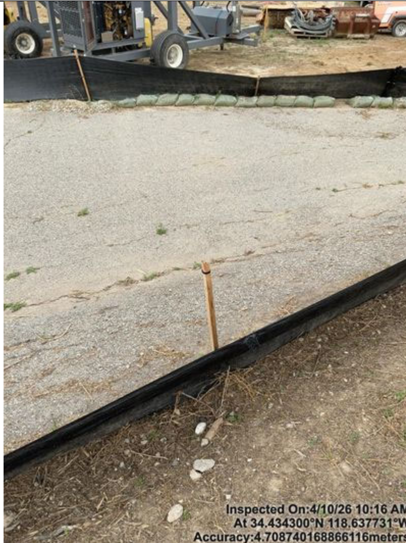
Photo 37 Silt fence detached from stake
