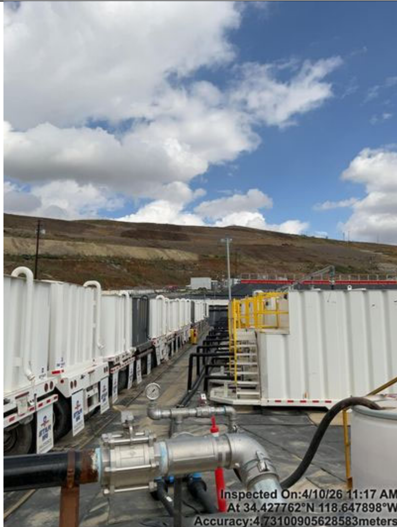
Photo 95 Treated leachate in tanks
