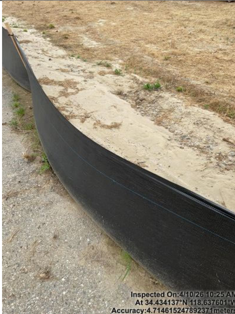
Photo 42 Silt fence bulge from sediment buildup
