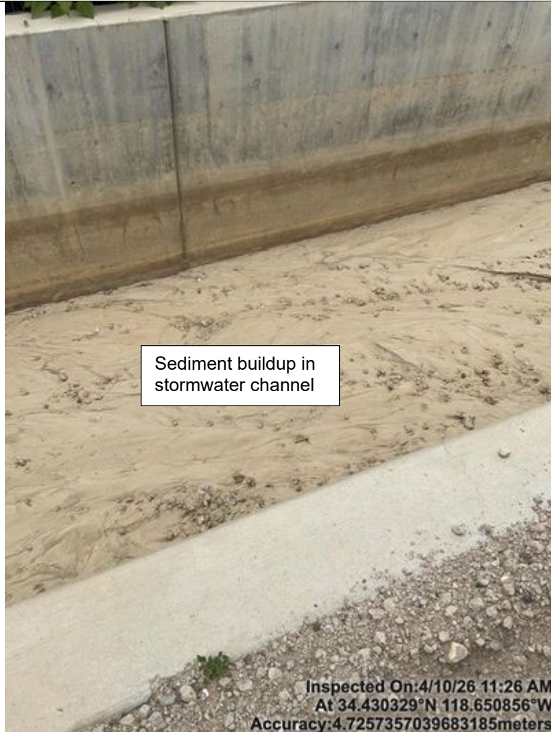
Photo 101 Sediment buildup in stormwater channel
