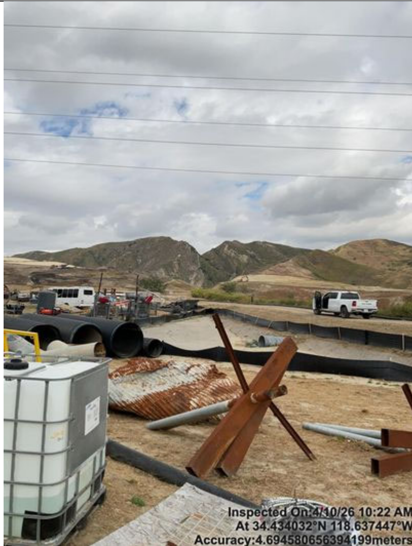
Photo 52 Equipment storage upgradient of the culvert
