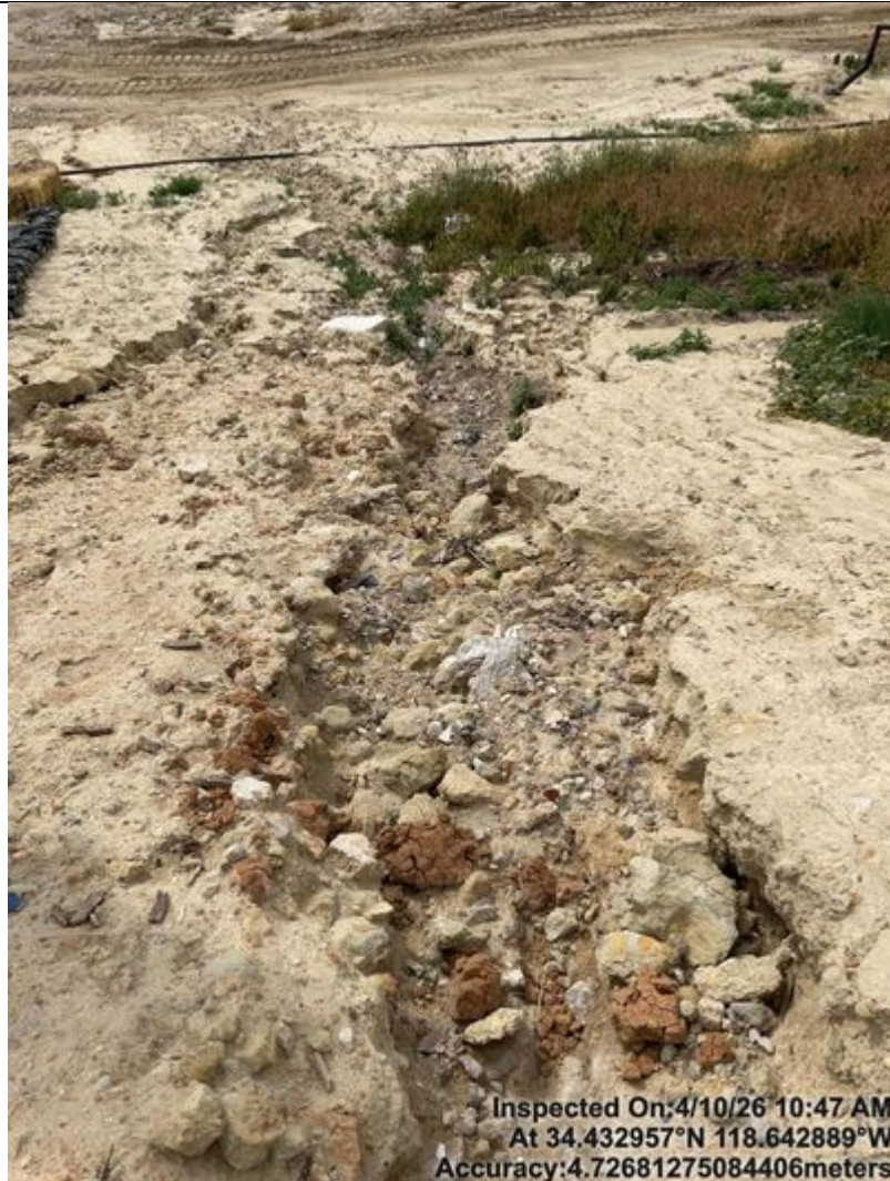
Photo 81 Close-up of erosion next to erosion control BMP
