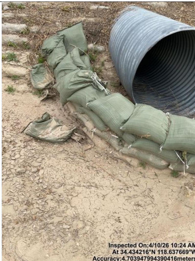
Photo 40 Sediment buildup around sandbags
