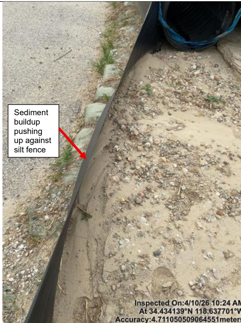
Photo 38 Sediment buildup along silt fence
