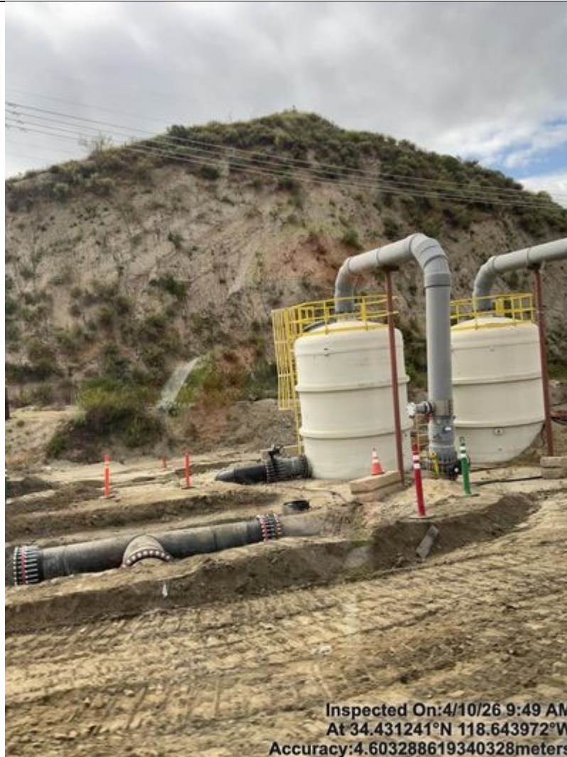
Photo 6 Air treatment vessels for H 2 S treatment
