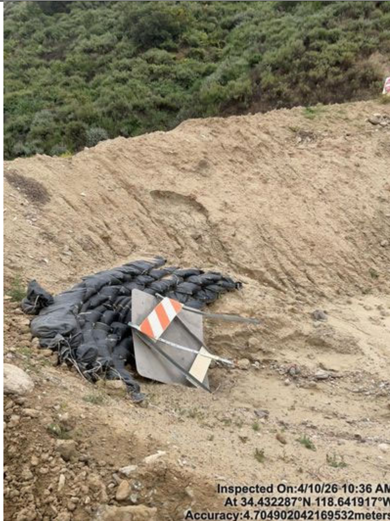
Photo 67 Fallen sign blocking the east inlet to the South Basin
