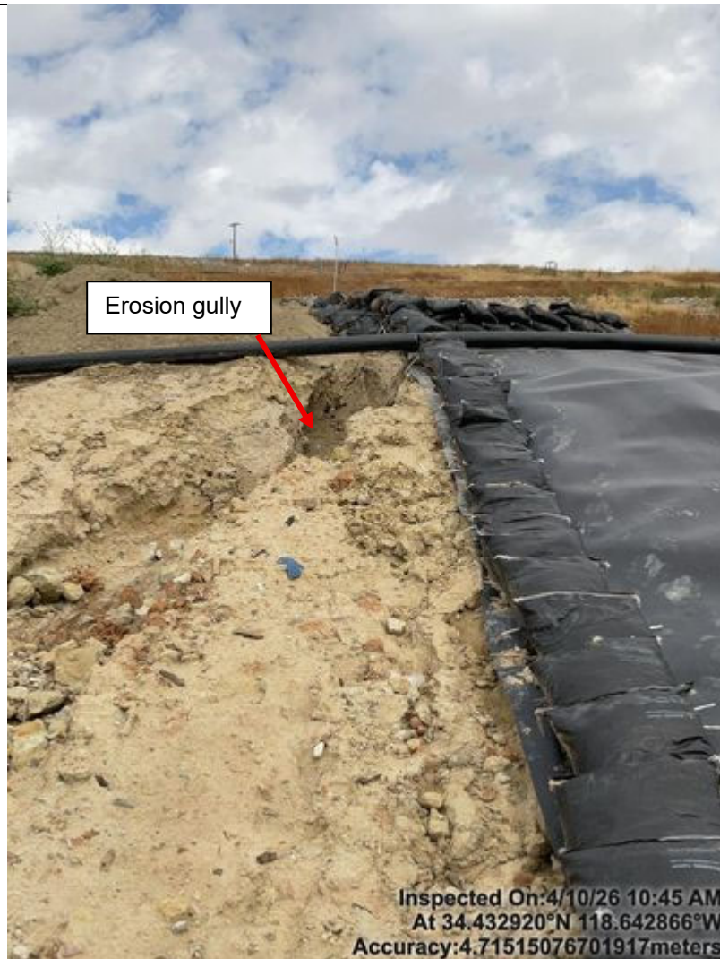
Photo 75 Close up of erosion gully next to the erosion control BMP
