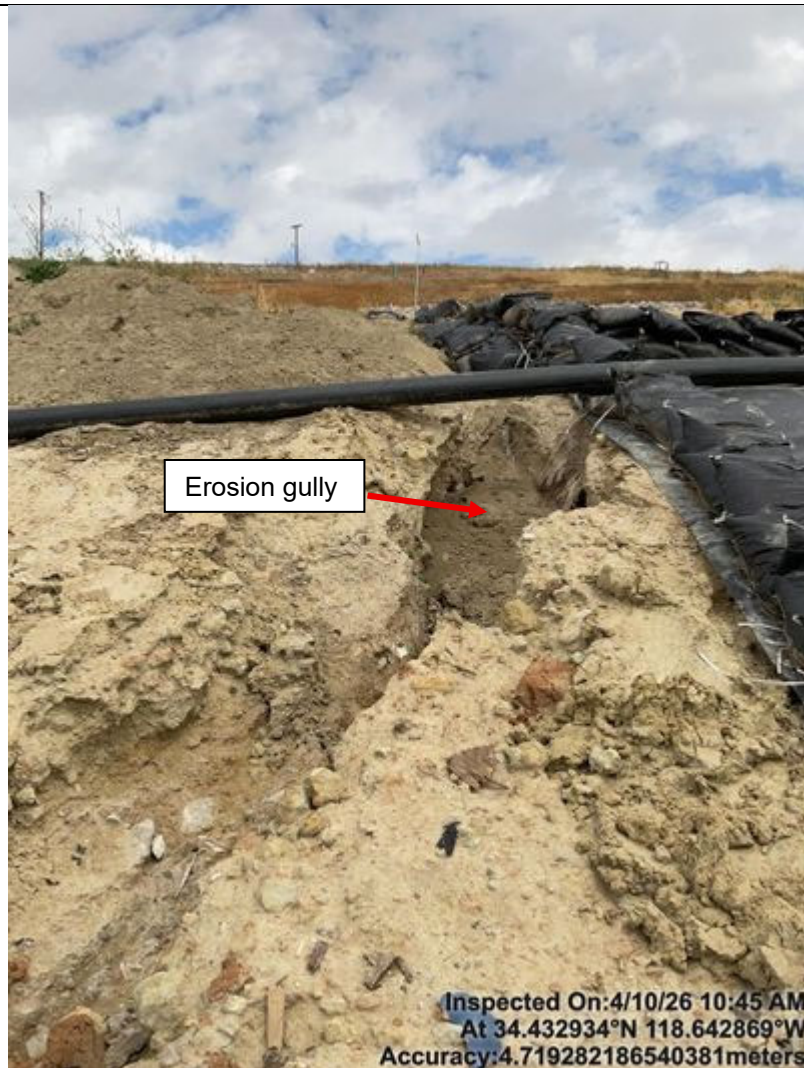
Photo 76 Close up of erosion gully next to the erosion control BMP
