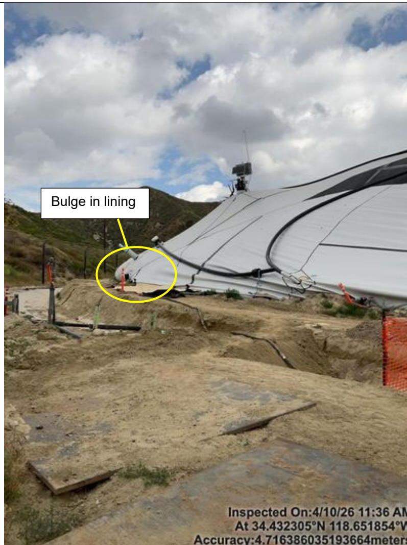
Photo 109 Another bulging area of west toe
