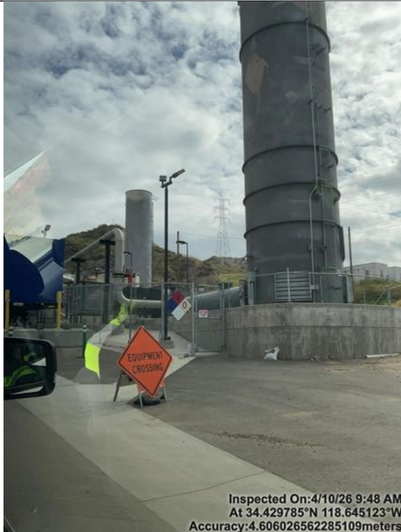
Photo 5 3 flares for gases burned from landfill emissions
