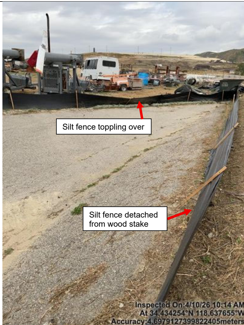
Photo 34 Silt fence with improper installation in need of repair.
