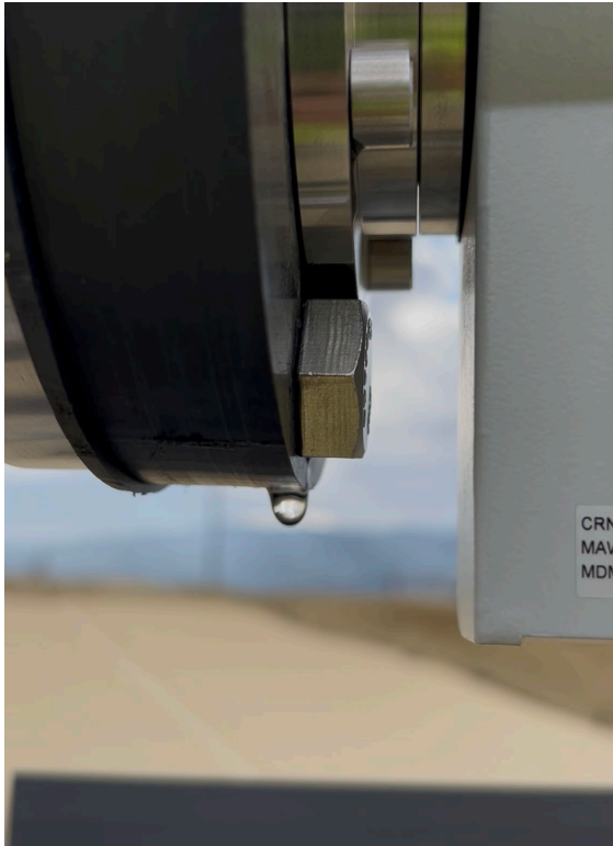
Pilot 4 - Liquid dripping from O2 flange
